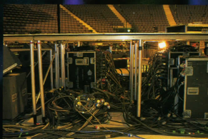
Behind the scenes - some of the cabling required
